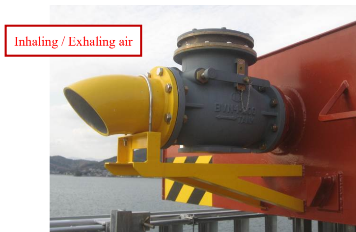
Photo 3) Safety device (Breather valve)
