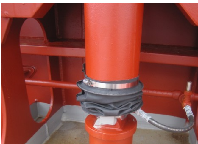
Photo 1) Bellows cover of the hydraulic cylinder for side-rolling hatch cover
